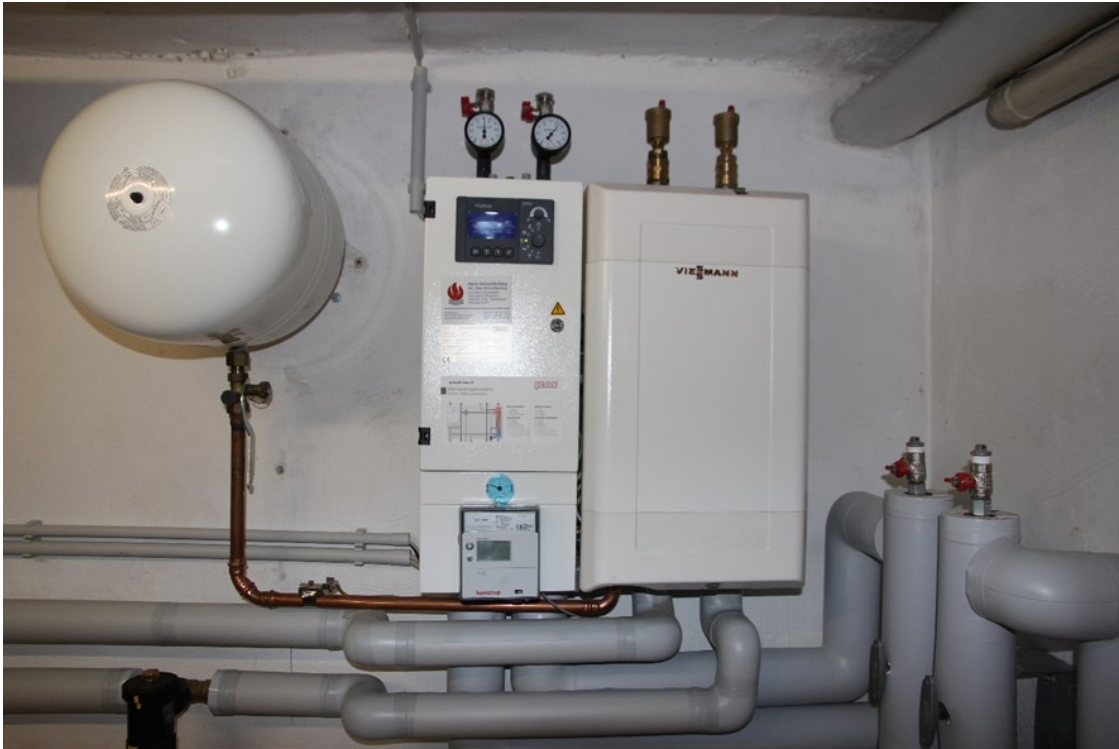
House transfer station. Source: Bioenergiegenossenschaft Mengsberg eG
