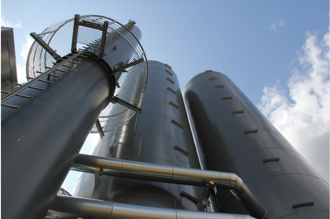
Buffer storage for solar energy. Source: Bioenergiegenossenschaft Mengersberg eG
