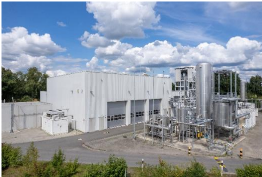
E-gas plant in Werlte, Germany (Figure: e-gas GmbH)
