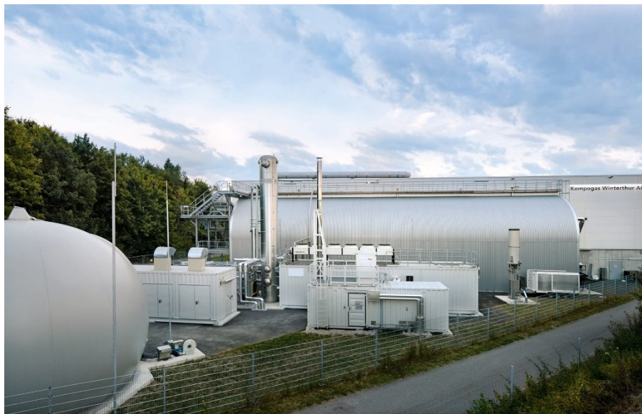
Figure 2: Gas upgrading plant, Winterthur, Switzerland (source: Hitachi Zosen Inova AG)
